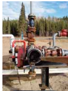
Pipeline Inspection Gauges, known as PIGs, are one of the final safety procedures used to ensure secure pipelines.
